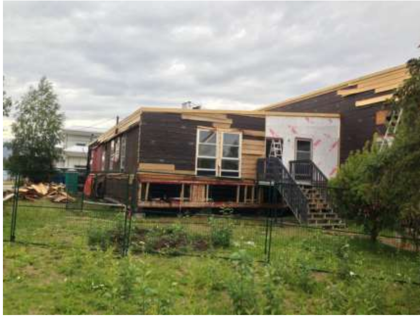
Rear view of the demolition under way. Photo courtesy Dan Davidson uffish@northwestel.net (In Dawson)
