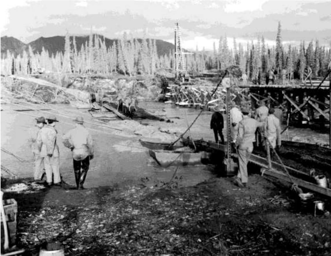
American army engineers struggle to keep a temporary pontoon bridge afloat (centre) while constructing a more substantial timber bridge (right). Do you have any memories of traveling or living on the Alaska Highway in the early days that you would like to share?" Credit: Yukon Archives, R.A. Cartter fonds, #1477.
