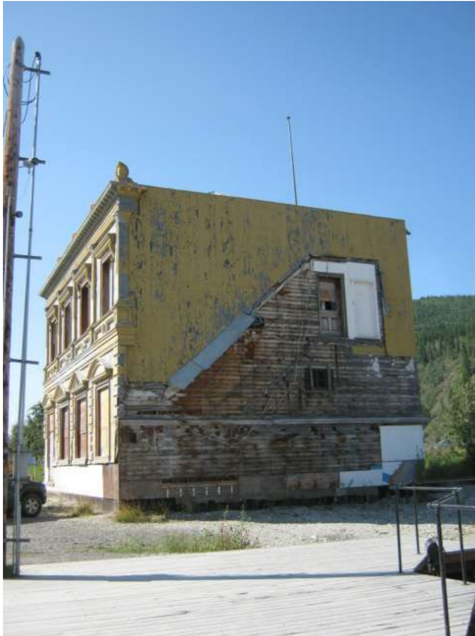
Tin siding is missing from the north side of the old CIBC Building where there was once an exterior stairway leading to the second floor.
