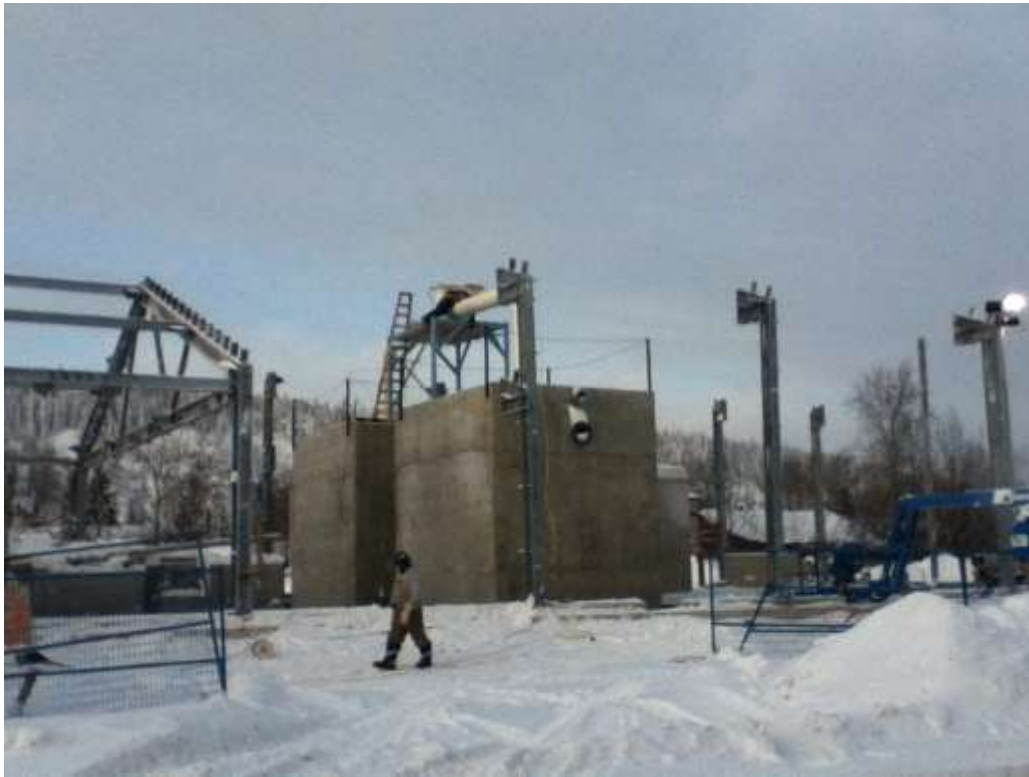
A worker can be seen hanging over the pipes that connect to the two vertical treatment shafts. There are two shafts to provide redundancy at the plant in case one should fail or require maintenance. Photo courtesy Dan Davidson uffish@northwestel.net (In Dawson)
