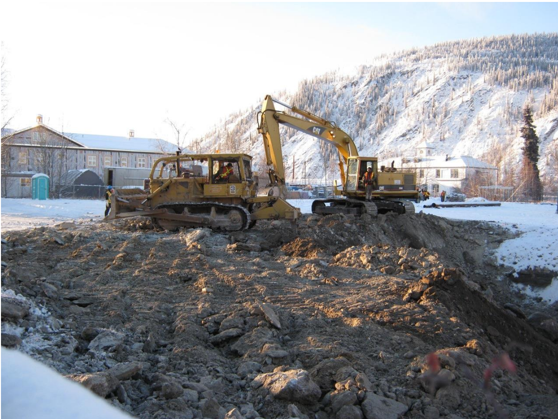
Corix Water Systems is continuing work on foundation excavation for Dawson's secondary sewage treatment plant, while keeping an eye out for coffins.
