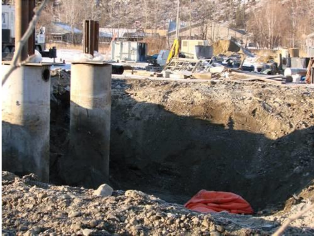
This pit was excavated around the Vertreat (vertical treatment) shafts. Photo courtesy Dan Davidson uffish@northwestel.net (In Dawson)
