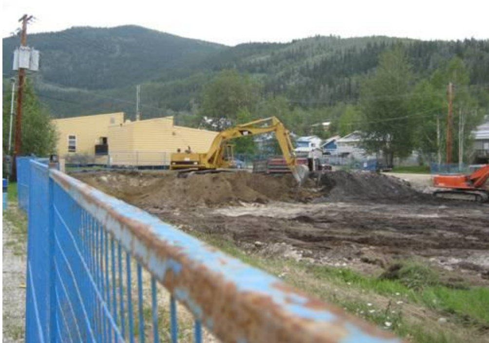
Foundation excavation begins on the new Dawson hospital . Photo courtesy Dan Davidson uffish@northwestel.net (In Dawson)
