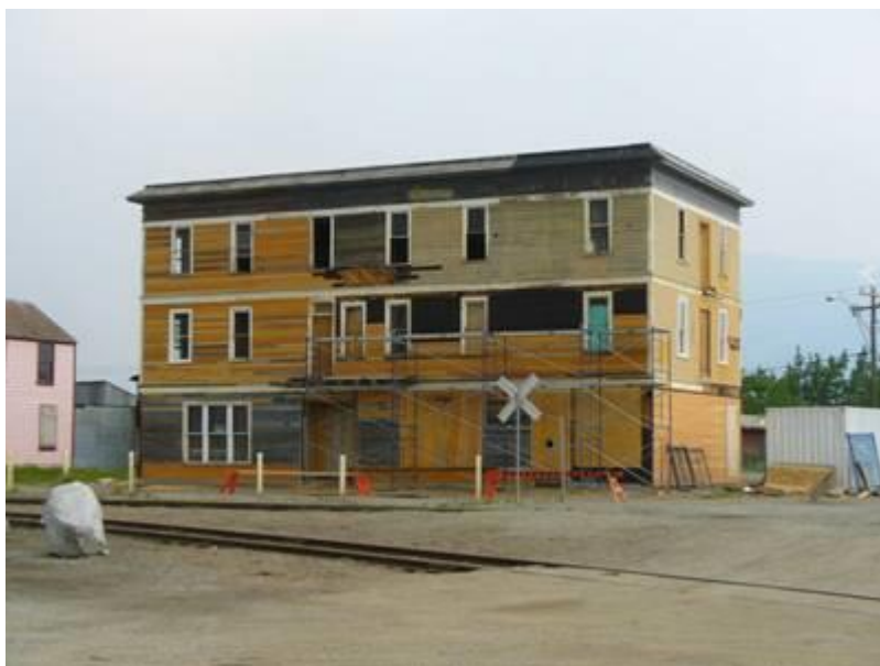
The old hotel in Carcross is undergoing renovations Photo courtesy Bev Buckway balc*northwestel.net (In Whitehorse)
