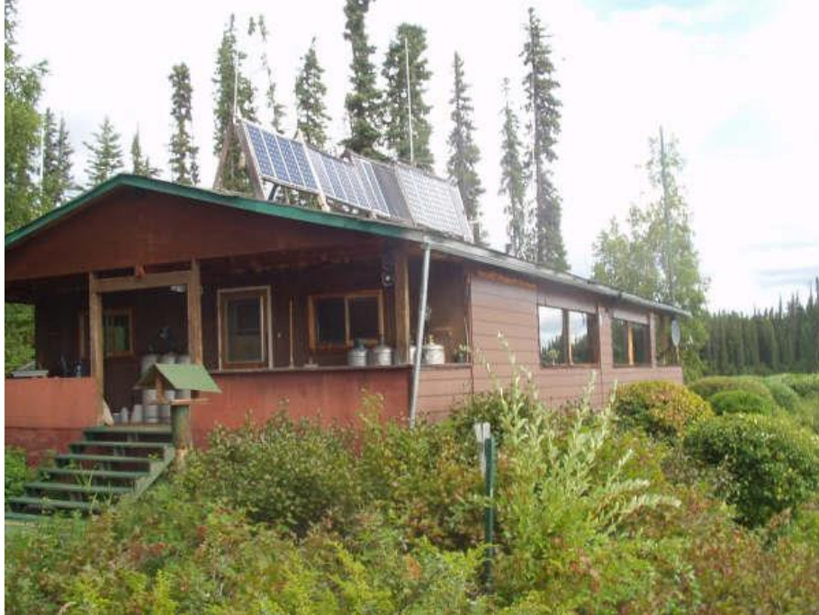
Solar power – Don Taylors Place at Stewart Lake
