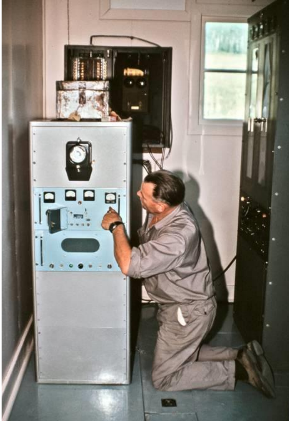
Out along the Yukon Network - Technician Ed Kerry making adjustments to a one of the McCurdy 40Watt RRT2 Low Power Relay Transmitters (LPRTs) serving the Yukon Network - Dawson City - 1963 Photo courtesy Tim Kinvig kinvig@northwestel.net (In Whitehorse)
