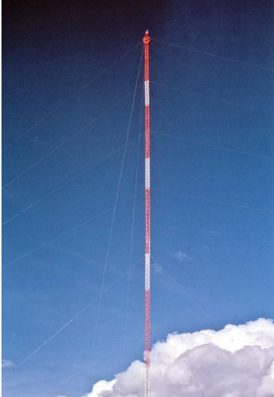
Installation of the CFWH transmitter site - Antenna installation - 2 riggers on top of the 286' tower.1962 Photo courtesy Tim Kinvig kinvig@northwestel.net (In Whitehorse)
