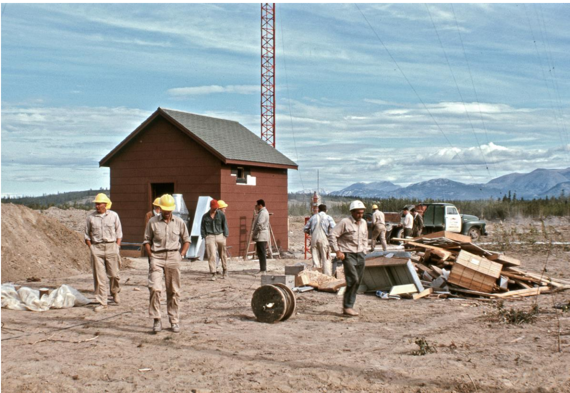
Installation of the CFWH transmitter site - 1962 Photo courtesy Tim Kinvig kinvig*northwestel.net (In Whitehorse)
