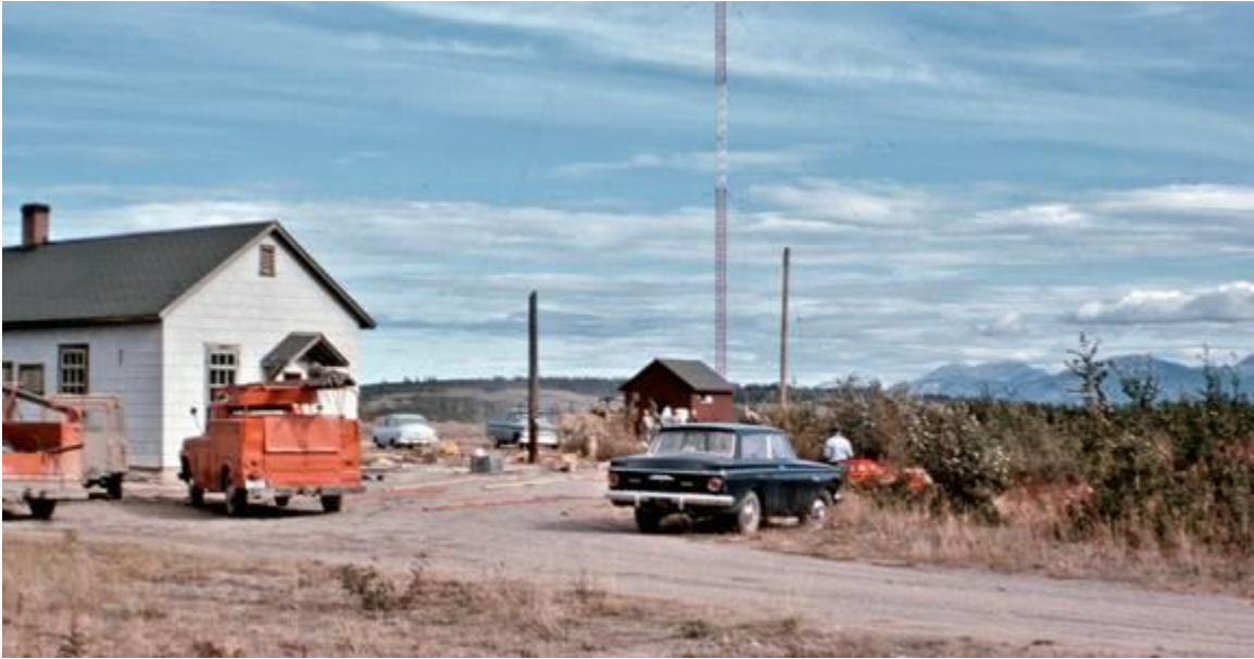
Installation of the CFWH transmitter site - 1962 Photo courtesy Tim Kinvig kinvig*northwestel.net (In Whitehorse)
