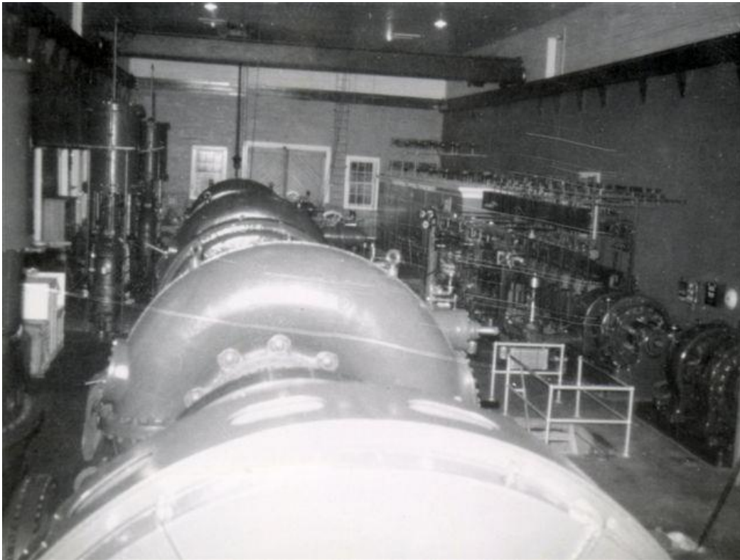
Inside Power Plant
