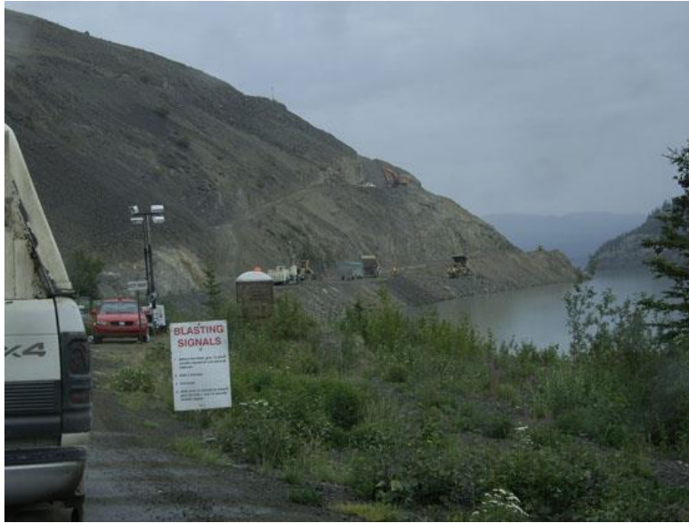
Road construction in full swing at the toe of Sheep Mountain along Kluane Lake on July 27/07.
