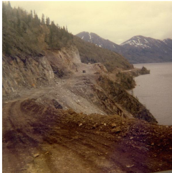
Photo of the haul road freshly blasted out of the rock along Tutshi Lake looking east.
