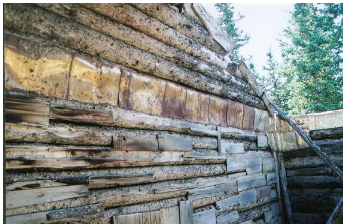
Notice the cans lining the wall under where the roof joins
