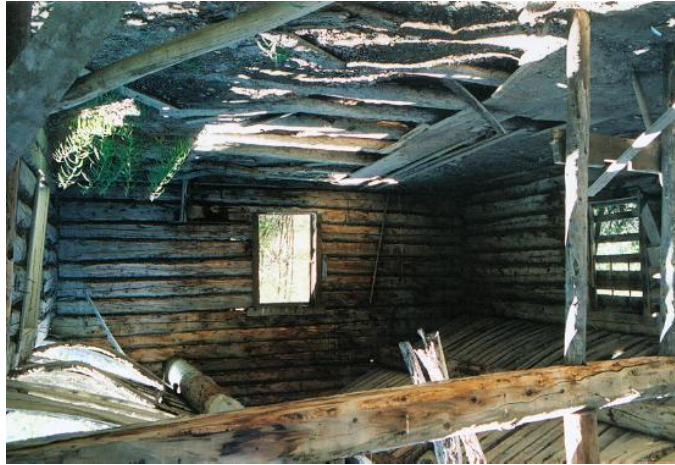
Collapsed Roof on large cabin
