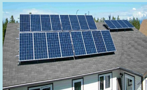
Solar panels on a rooftop. Credit: John Maissan.
