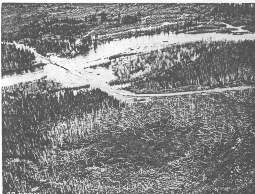
Fig. 25 - Flood of bridge approach - McQuesten River May 23, 1957.
