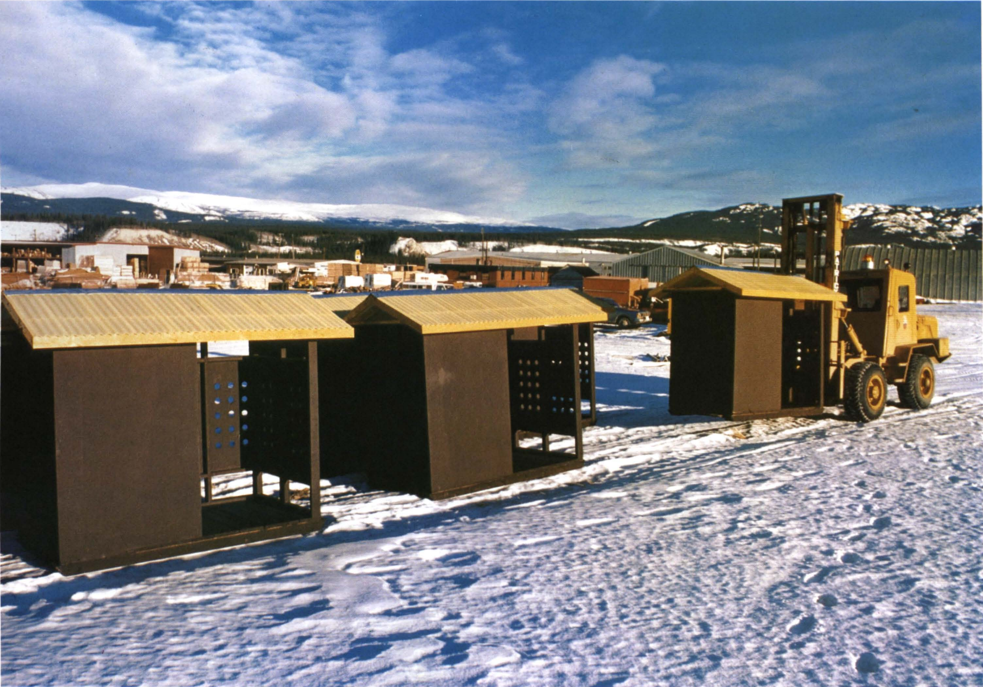
Inmates of the Whitehorse Correctional Institute assist the Parks and Historic Sites Division in the construction of campground facilities.
