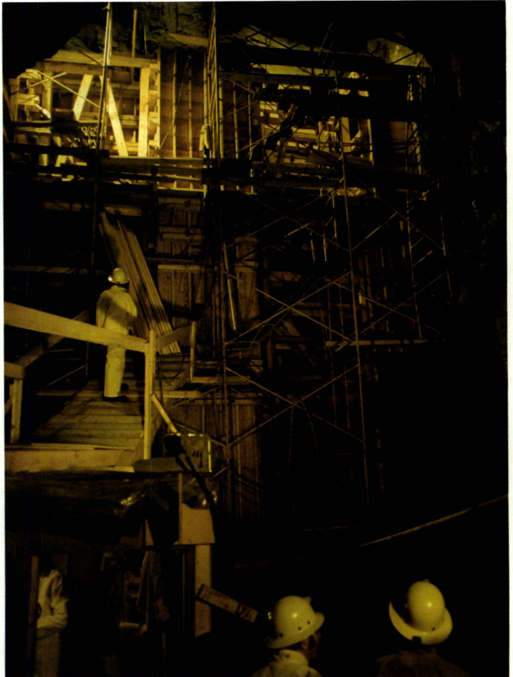
Work progresses underground at the Aishihik Power Project. When completed, the new site will produce 30 megawatts of power.
