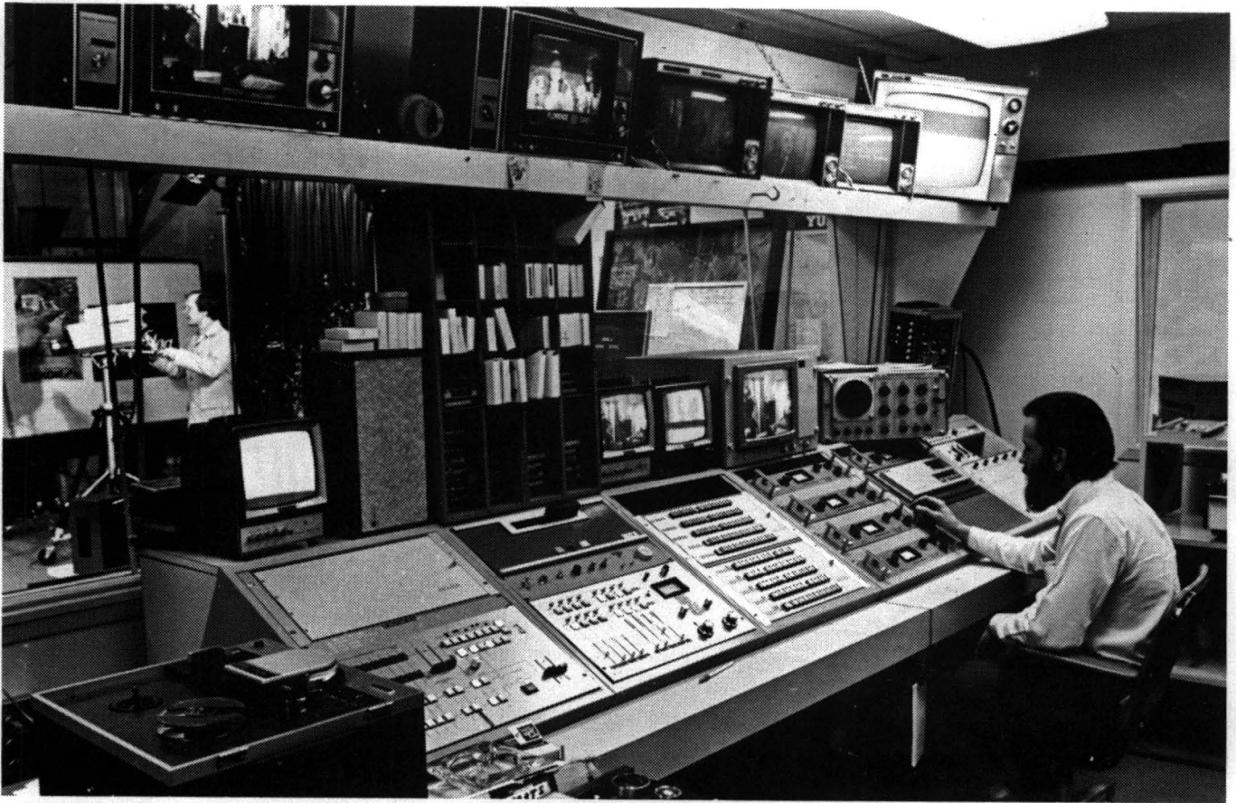
The cable television facilities in Whitehorse provide the capital city with a number of colour services.
