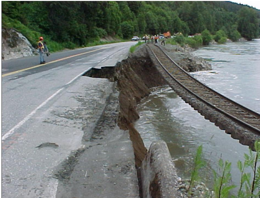
Picture 23: Inadequate Erosion Protection
