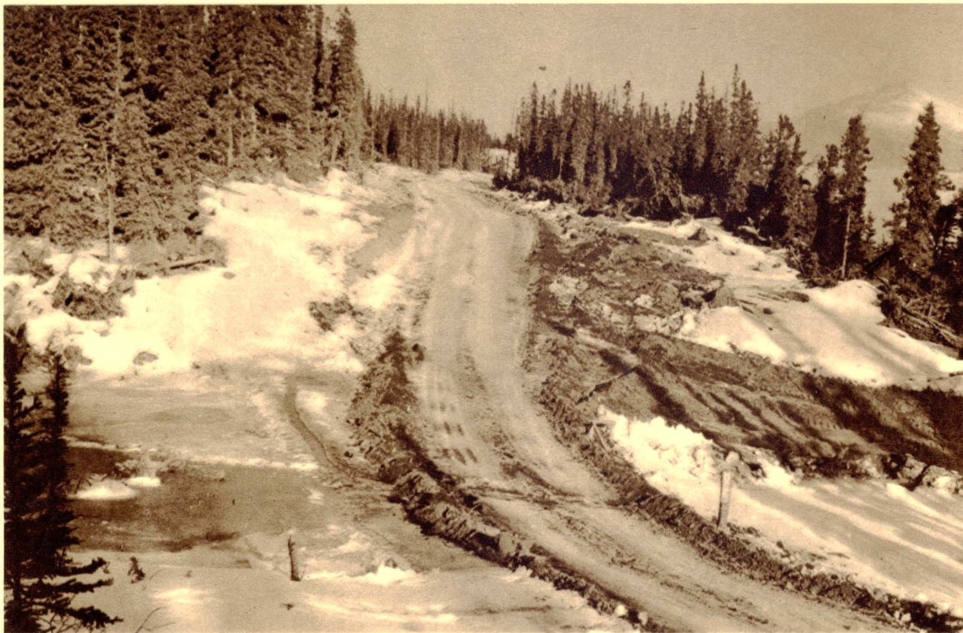
FROZEN DIRT PLACED ON THE SECTION OF THE ALASKA HIGHWAY TO LESSEN ICE HAZARDS
