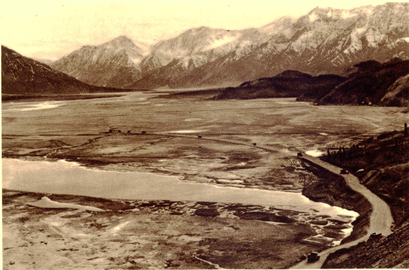
BUILDING THE ALASKA HIGHWAY ACROSS 1½ MILES OF SILT FLATS AT THE MOUTH OF THE SLIMS RIVER AT KLUANE LAKE ABOUT 160 MILES WEST OF WHITEHORSE
