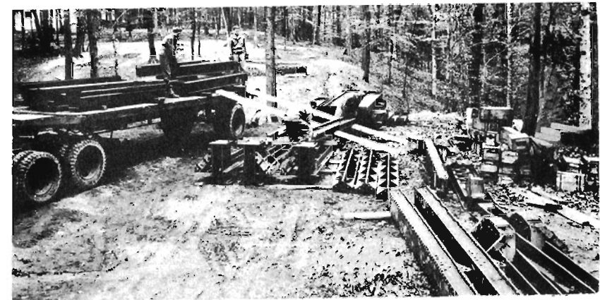
Figure 40. Unloading light steel sections from a trailer by hand. Skids are used to slide beams to the ground.
