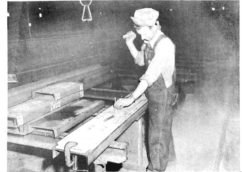
Figure 44. Wood template used to guide center-punching for holes in a short steel channel.
