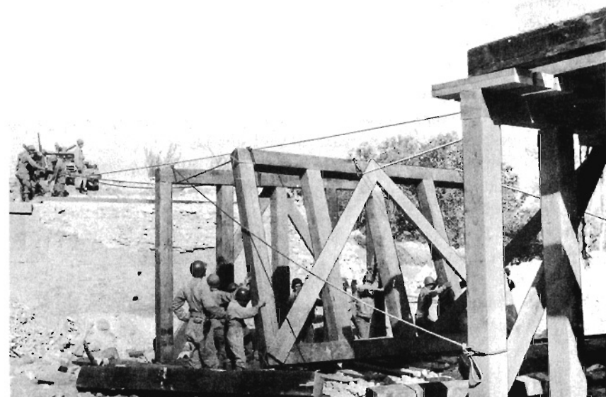
Figure 125. Raising framed bents into position with truck winch. Bridge details are not standard.
