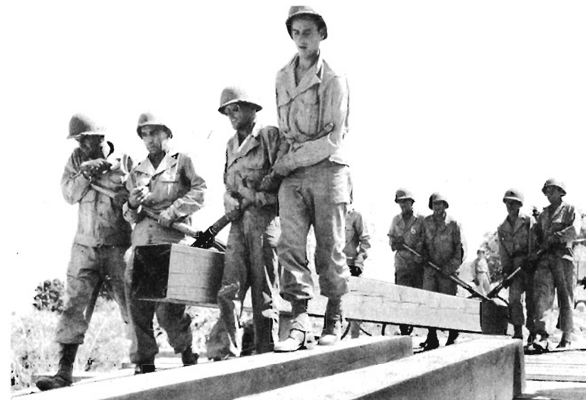
Figure 126. Bringing up timbers to be set in place with erection equipment. Heavy timbers are being manhandled with peavies.
