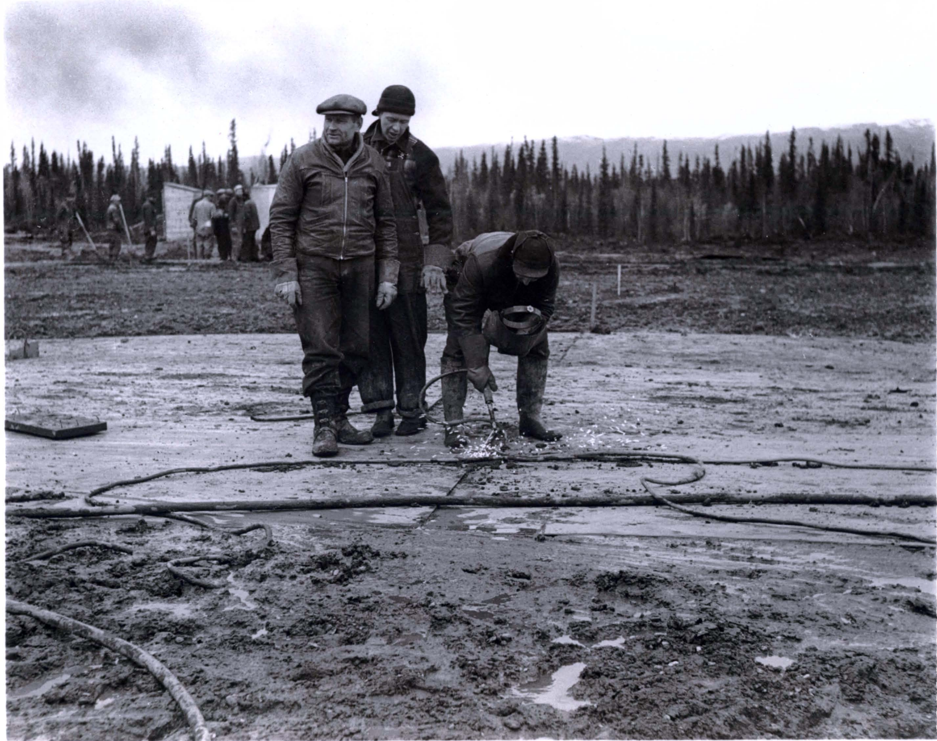
First welding on the first 80,000-barrel Constructor's storage tank, Norman Wells, September 23, 1942.
