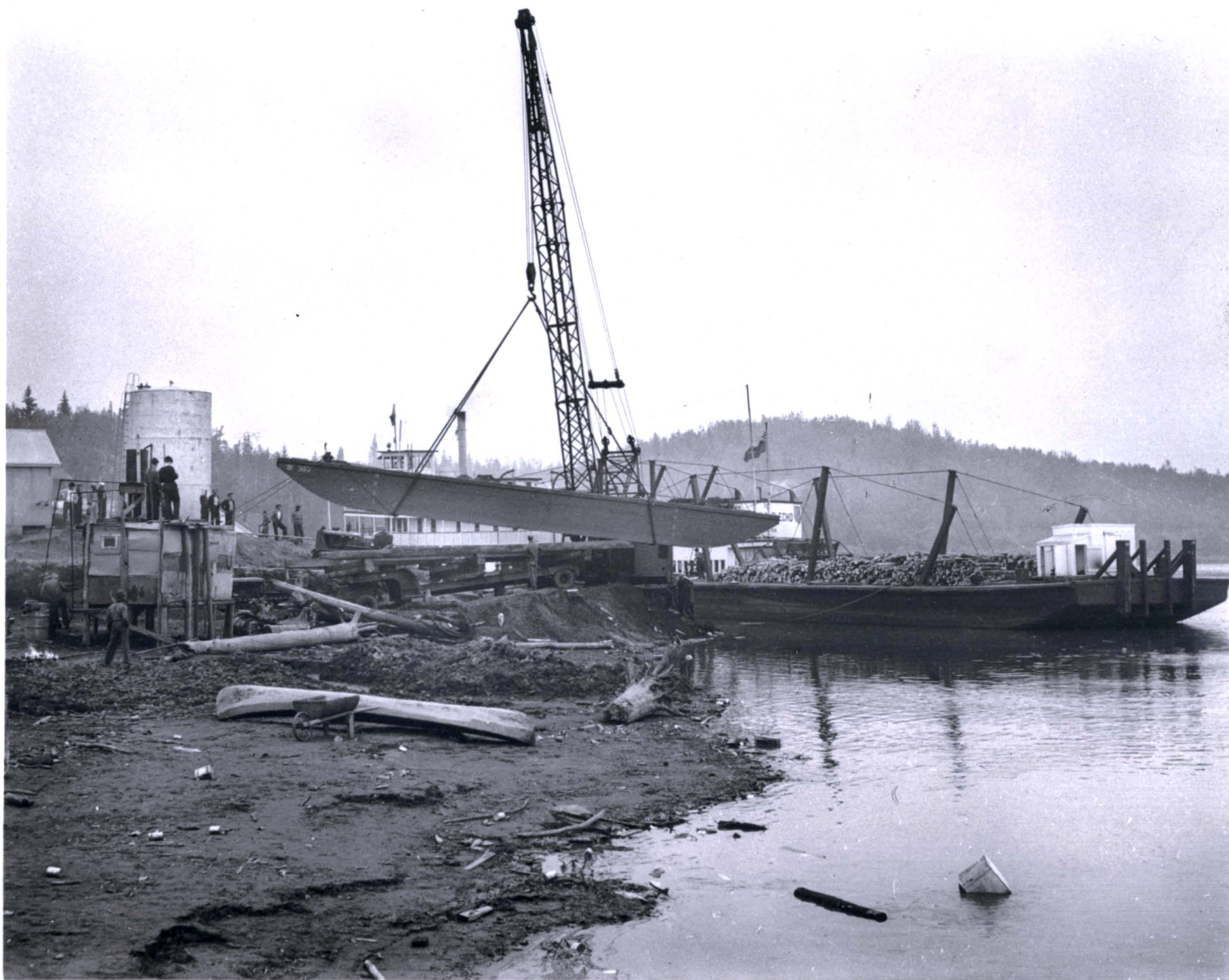
Barge being lifted out of water at Fitzgerald and placed on the trailer for portage haul.
