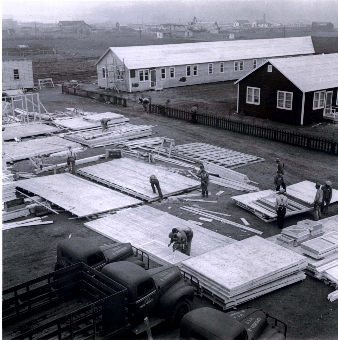
Crew quarters being fabricated at Camp Prairie for shipment to airfield sites and Camp Canol.
