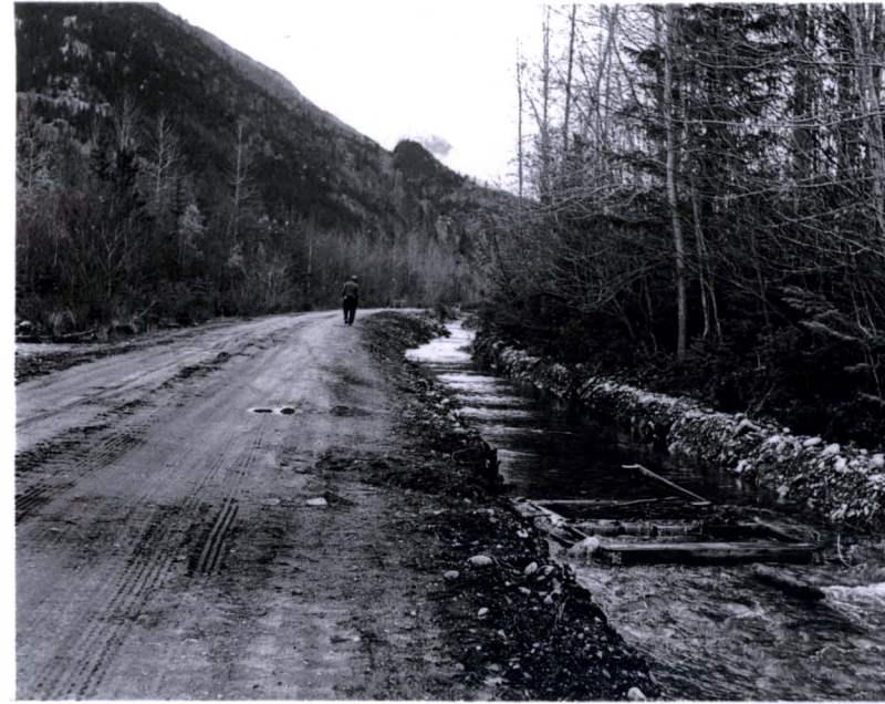
Skagway—Constructor's road. The creek diverts a hillside stream from the tank sites.
