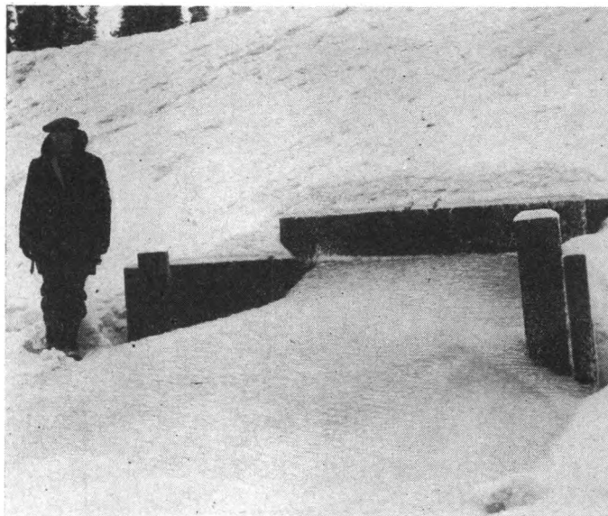
OUTLET OF A CULVERT THAT IS COMPLETELY FILLED WITH ICE.
