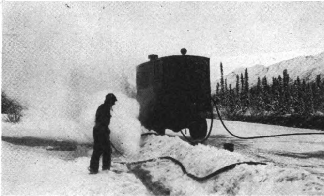
THE STEAM GENERATOR IN ACTION.
