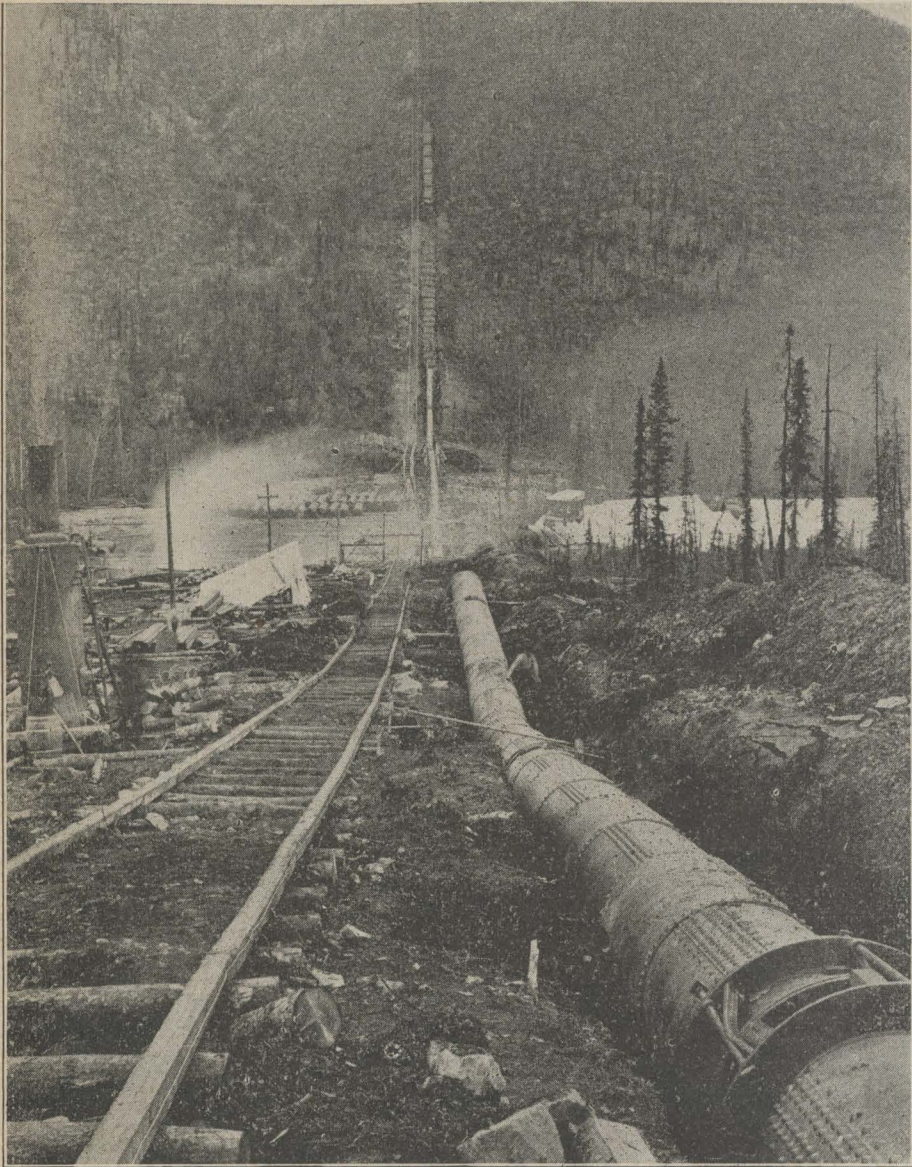
A Section of Pipe Line.
