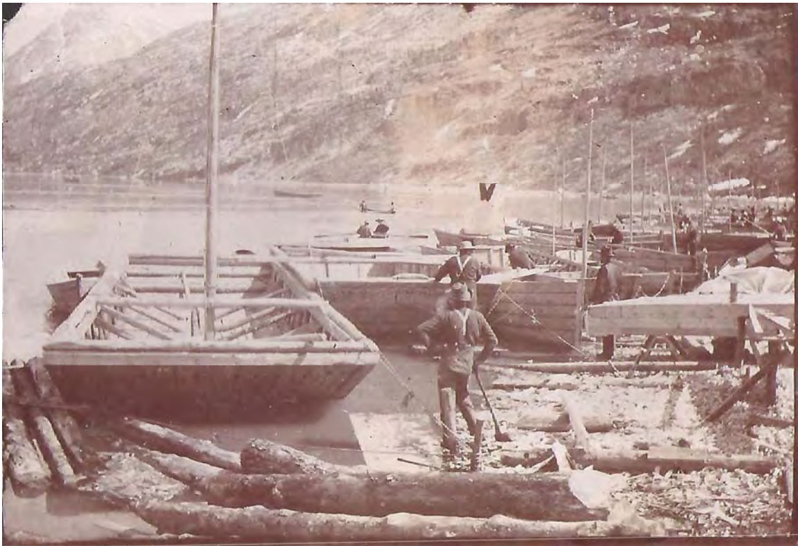
FIGURE 2.5. Scows on the water and being constructed on land at Bennett (Goddard collection, courtesy of Fay Goddard).
