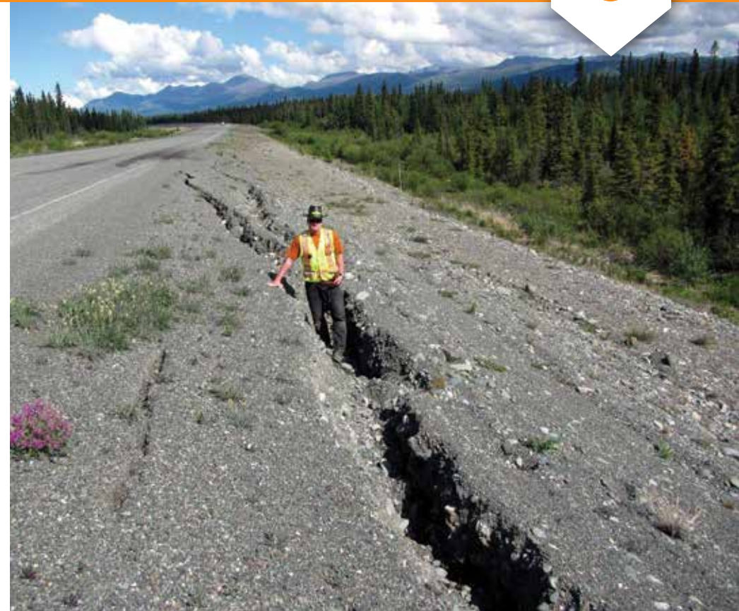
Road damage from the thawing of permafrost.
