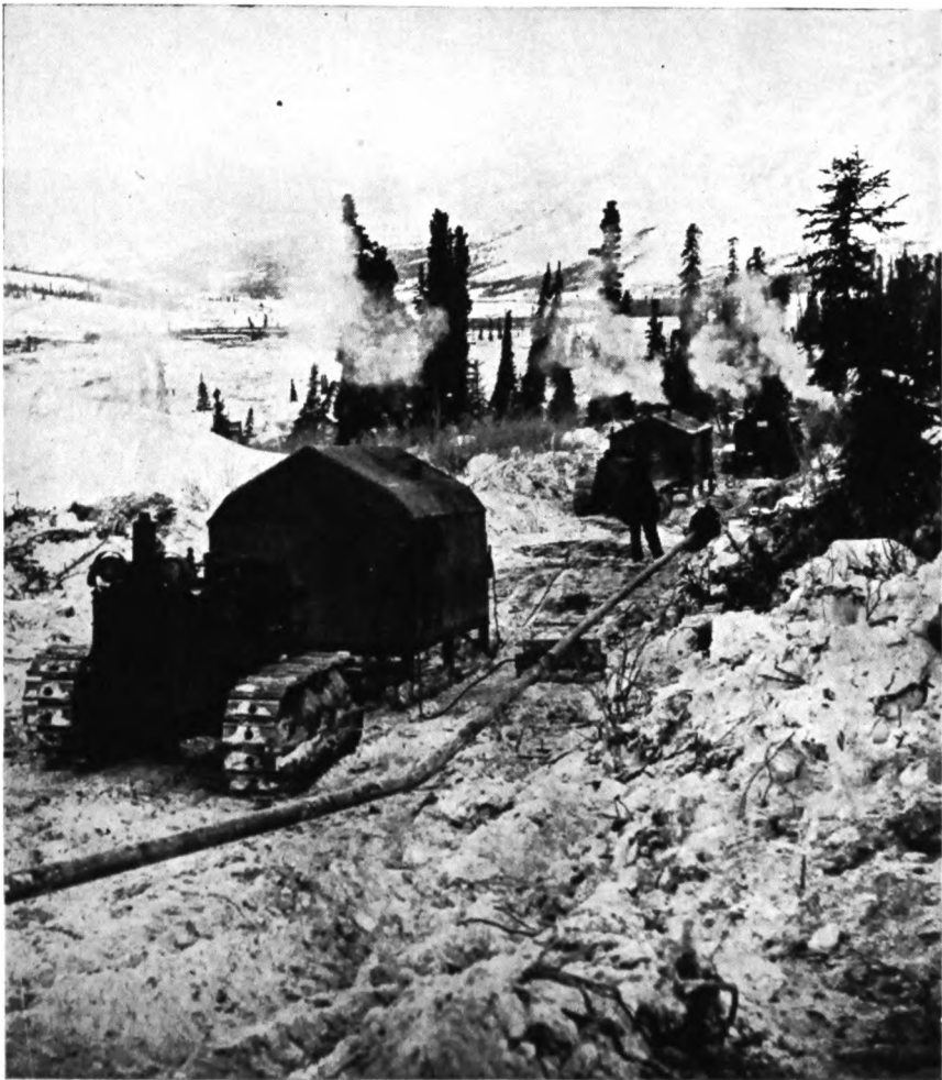
The two lines nosed together for the final weld on February 16th.
