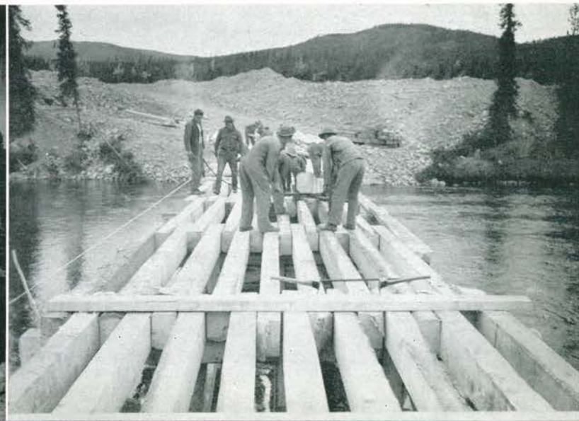
Stringers, cut from big spruce logs, are being laid by husky soldiers at the Rancharia, mile 119.
