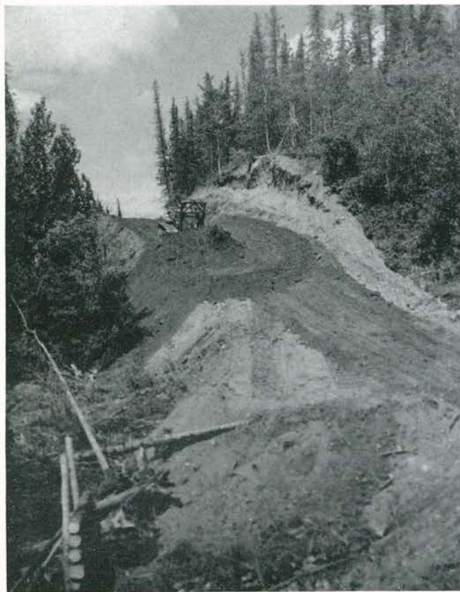
A dozer busy in a cut-and-fill job. An abundance of gravel nearby made short work of many otherwise difficult spots.
