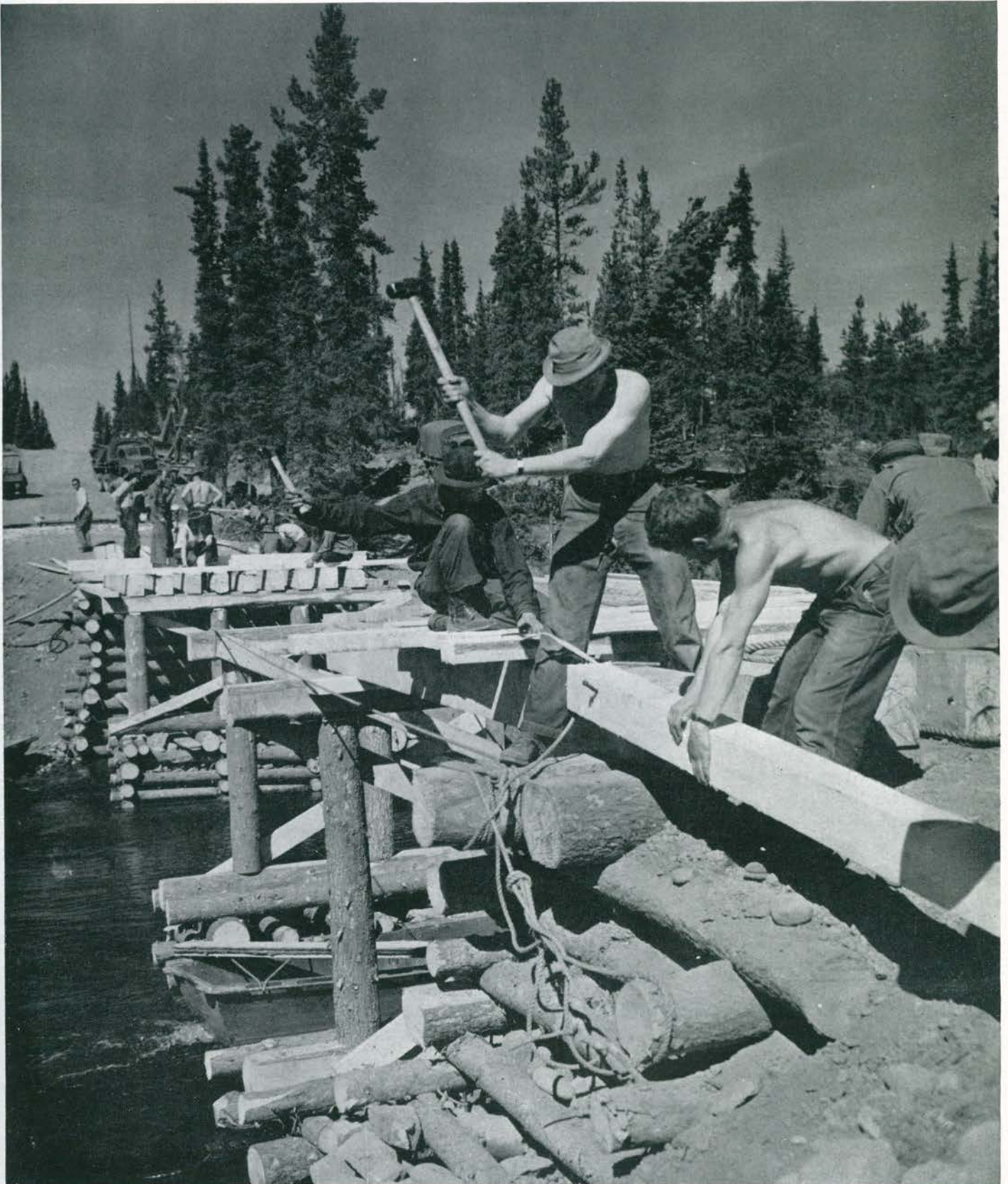
Multiple action nicely "frozen" is represented in this fine shot of the Morley River bridge under construction. Two newly completed sections of road will be joined by the bridge.
