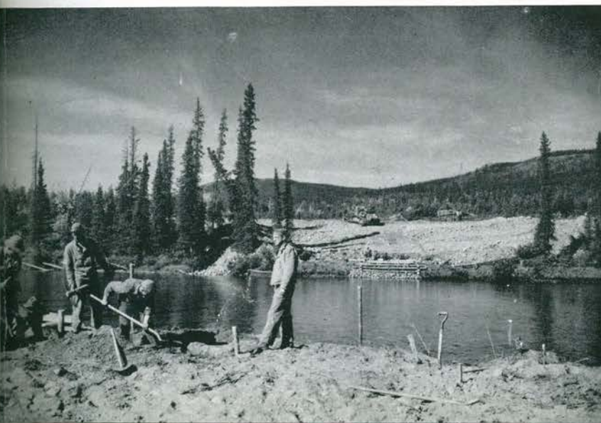
D Company, commanded by Capt. Walthall (in foreground), begins work on the bridge at the second crossing of the Rancharia river.
