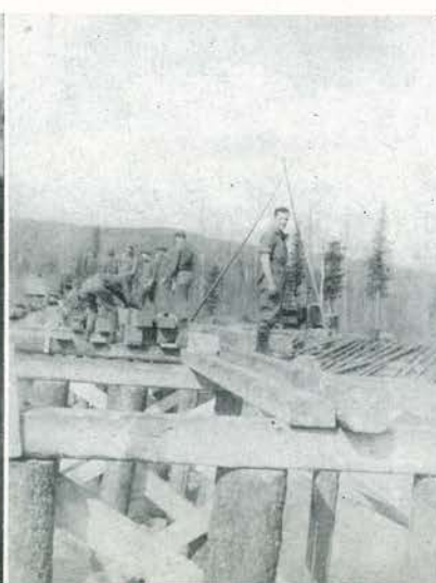
Stringers go down on log bents as C Company sets a fast pace.
