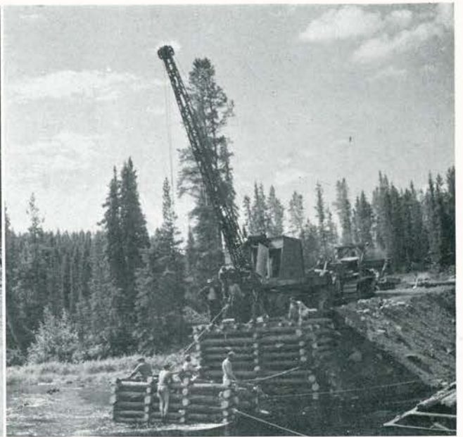
A mobile crane placing the footing for a trestle bent as D Company starts constructing the Morley River bridge at mile 26.
