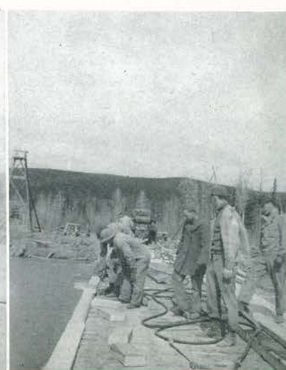
Nearing completion, the Tanana bridge is about ready for another battle with nature.
