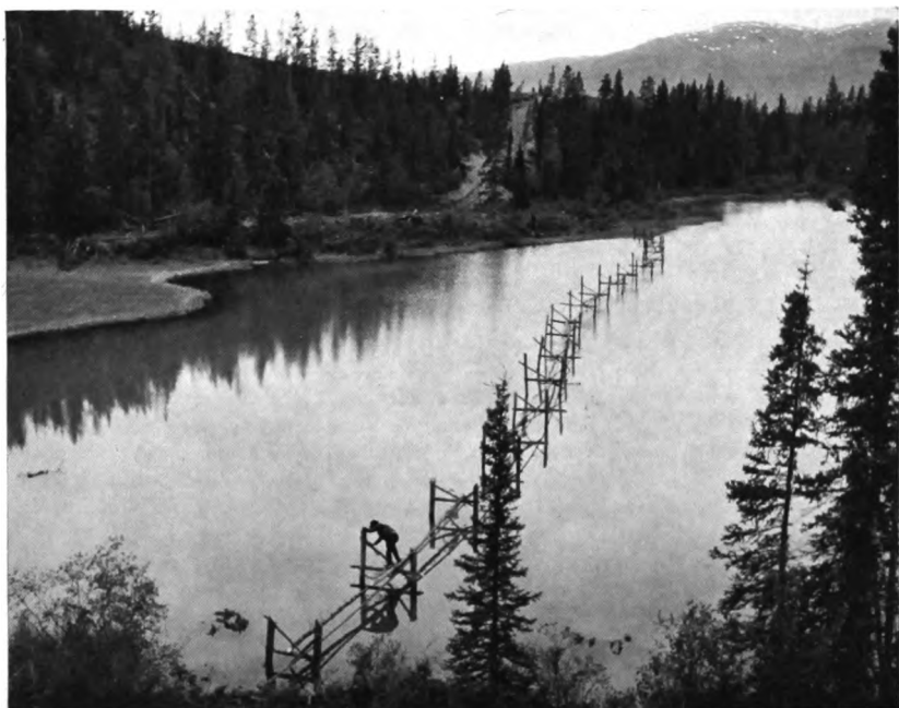
FIG. 12—A section of Canol pipe line being laid across a Yukon lake. (National Film Board.)
