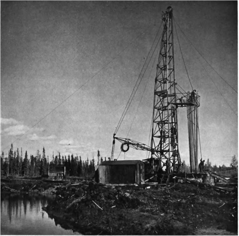
FIG. 18—Canadian drilling crew at work at Norman Wells; note the trenching to drain off water from the thawing muskeg. (National Film Board.)
