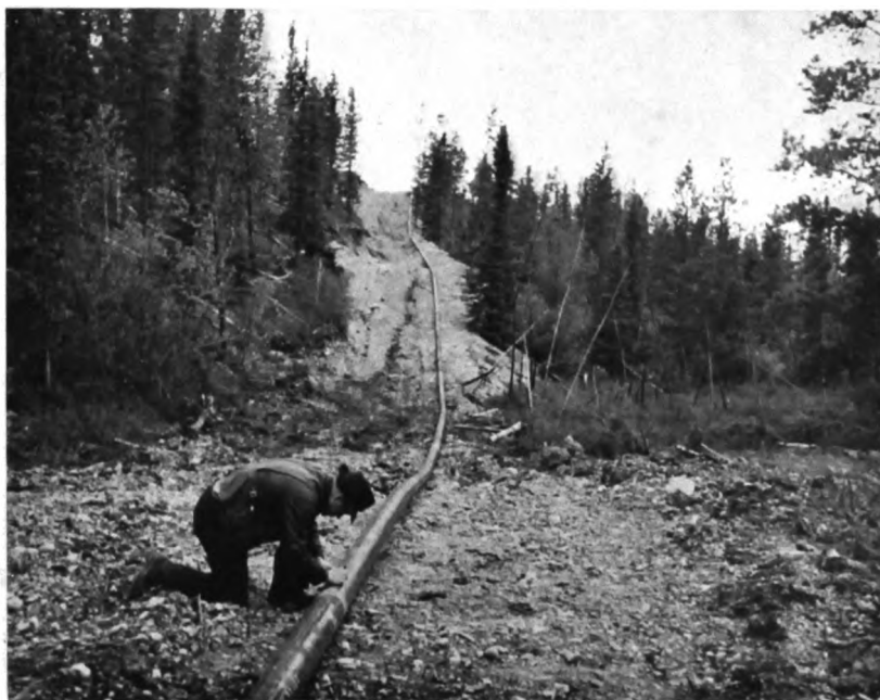
FIG. 14—Pipe line in position near the western end of the Canol route. A Texas oilman checks joint weldings. (National Film Board.)
