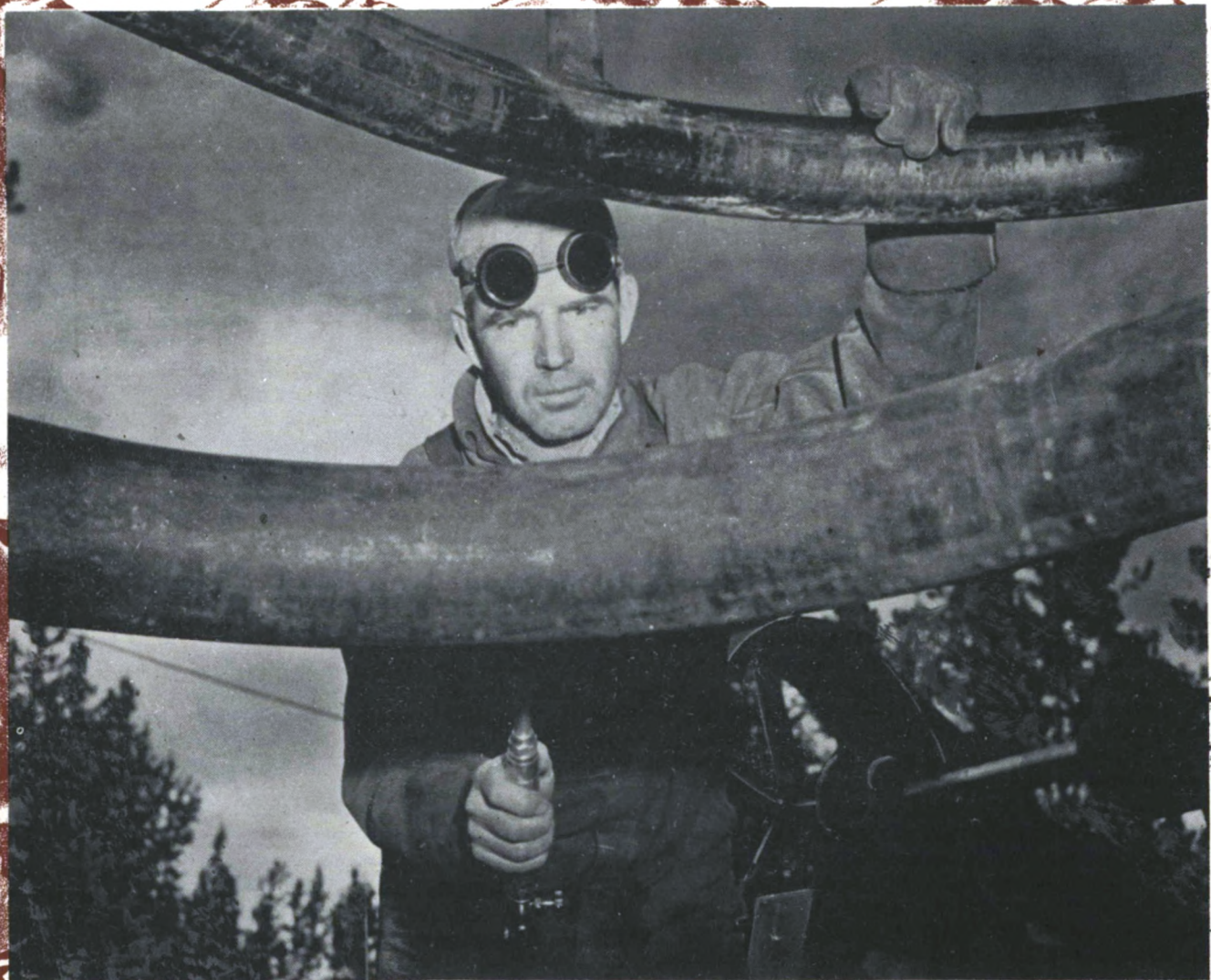
Harold "Denver" Atkins, Denver welder, applies welding torch to elbow of pipe made to allow for expansion and contraction of pipe from extreme heat to extreme cold.
