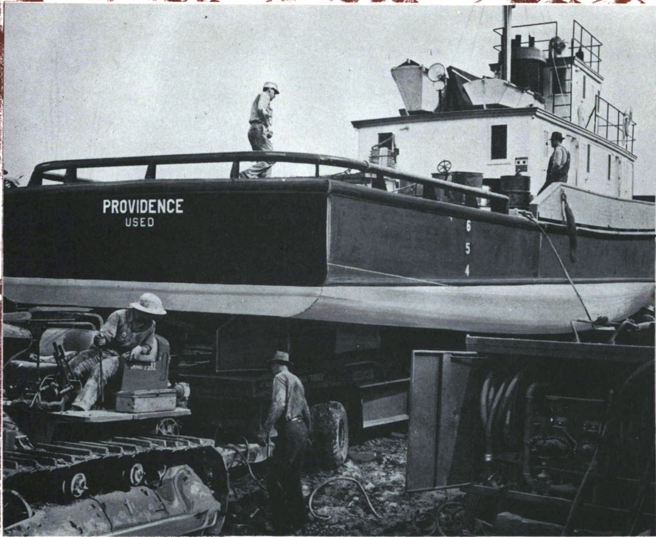
Tough hurdle is 16-mile portage around Pellican rapids at Fitzgerald and Fort Smith on N.W.T.-Alberta boundary. Here the 104-foot Providence, one of new steel tugs, is being towed across portage by caterpillars.
