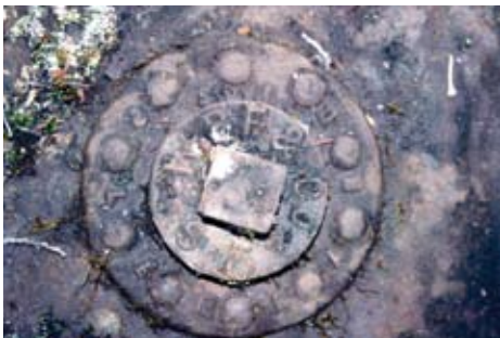
Manufacturer's mark, "WPF & Co. San Francisco," on boiler.
