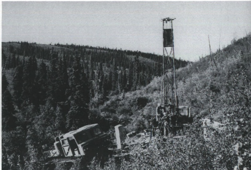
Rotary drill hole No. 3 intersects 175 feet of massive sulphides in No. 1 orebody.
