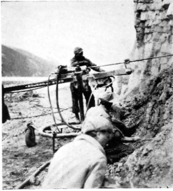
U.S. ARMY Engineers hacked their way through forest and mountain. With portable drills and jack hammers they cut a roadbed around Muncho Lake.
