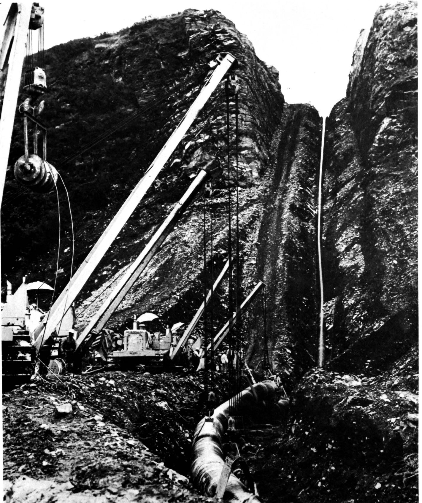
Pipe being lowered into trench on trans-Alaska oil pipeline. Similar techniques are proposed for natural gas pipeline construction (Alyeska)
