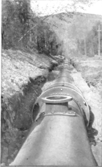
Portion of high pressure pipe line crossing Klondike Valley, showing man-hole and expansion joint.
